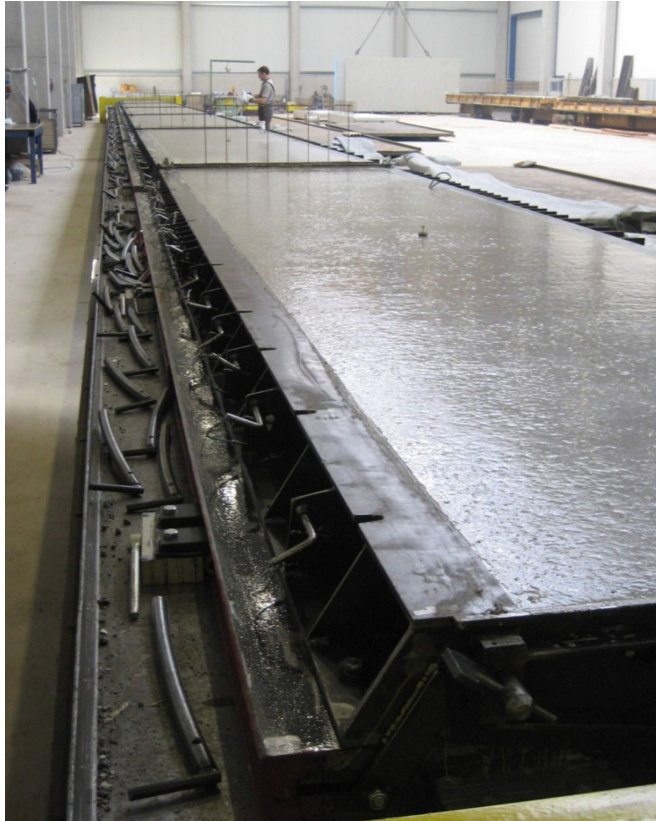
The tank construction in the US shortens transport routes, saves time and money, reduces carbon emissions, and supports the local job market. (Photo: Collins Precast)
