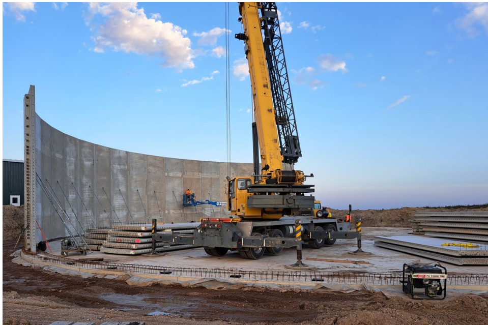
Together with Collins Precast, we can produce one Anaerobic Digestion tank per week with a net volume of approx. 2.2 million gallons. (Photo: Collins Precast)
